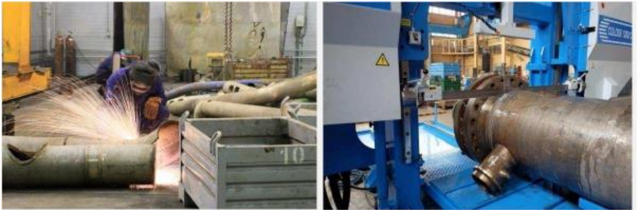
Figure 18. Cutting methods: hot cutting – plasma cutting, acetylene oxygen cutting; cold cutting – band saws, electric hand saws, electric and hydraulic shears, etc.
