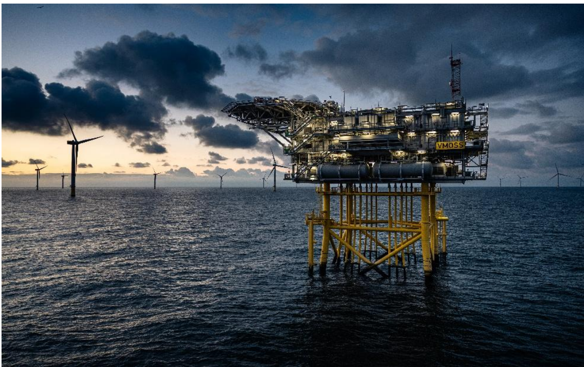
Figure 2.3.4.2. Offshore substation (Veja Mate (402 MW), Germany, developed by Copenhagen Infrastructure Partners (CIP))
