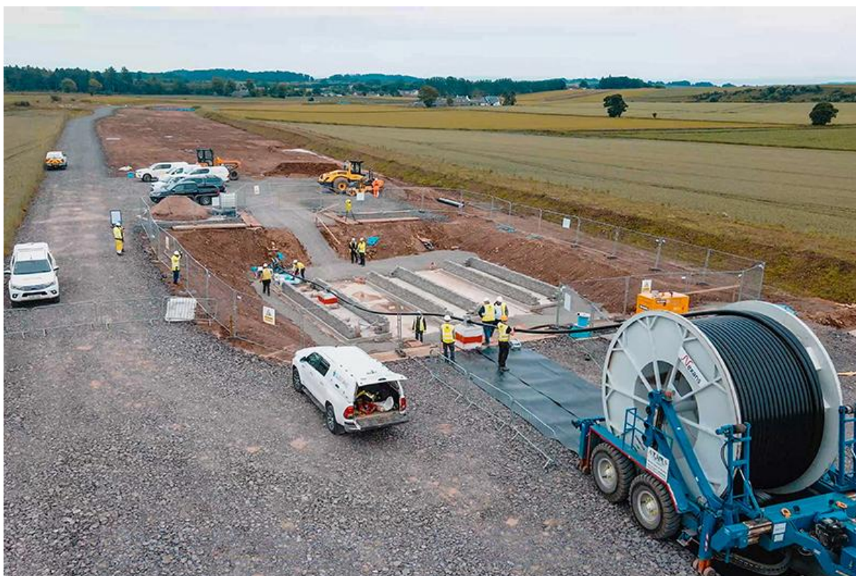
Figure 2.3.4.4. Transition Joint Bay (TJB) located close to landfall where offshore and onshore cables are connected. Source: SSE Renewables, Seagreen Offshore Wind Farm (1.1 GW), Scotland
