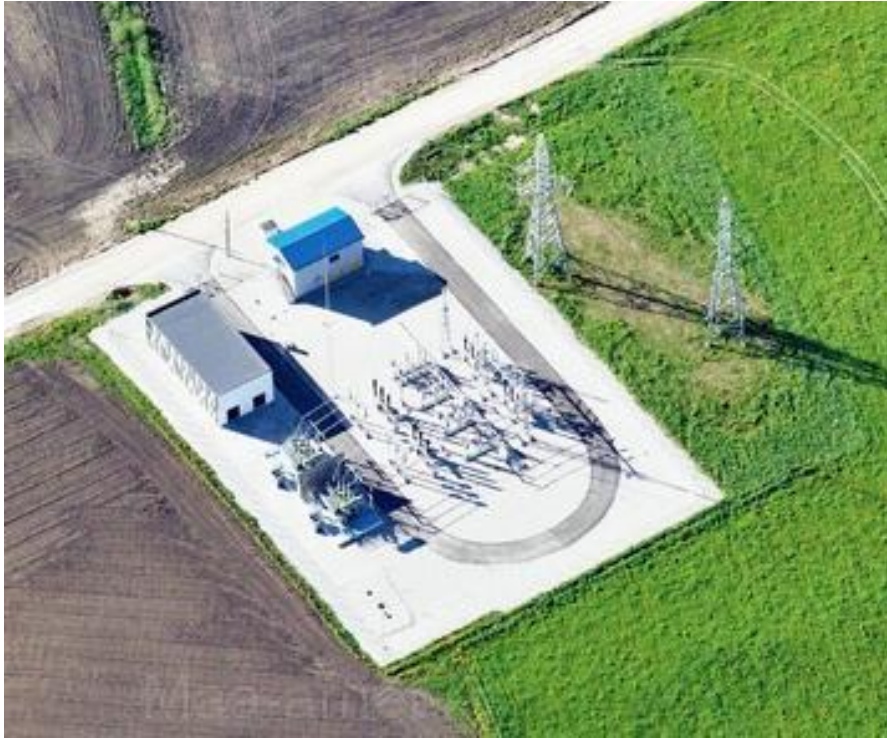
Figure6 . Illustration of a 110 kV substation – Järeda substation. Source: Land Board aerial photograph.
