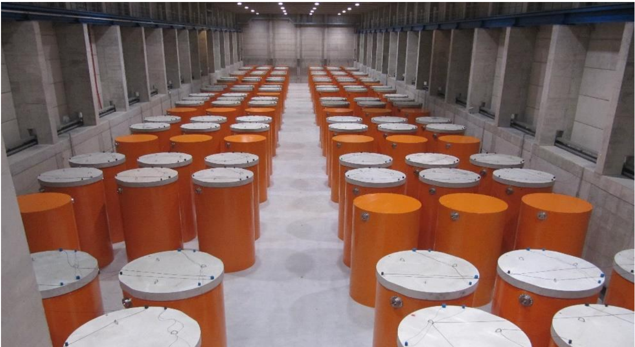
Figure 3.2-3. Cask storage hall of the SNF storage facility ISFSF-2
