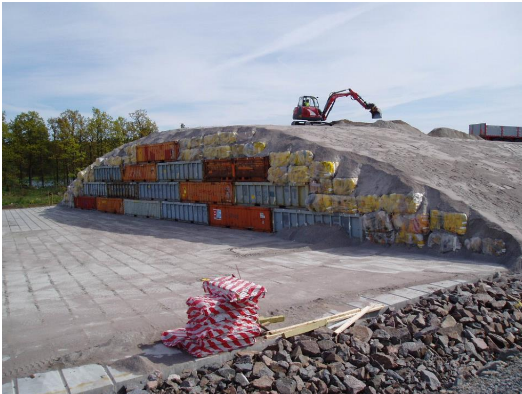
Figure 3.2-28. The structure of the VLLW repository module consists of waste packages and the formation of protective engineering barriers covering it
