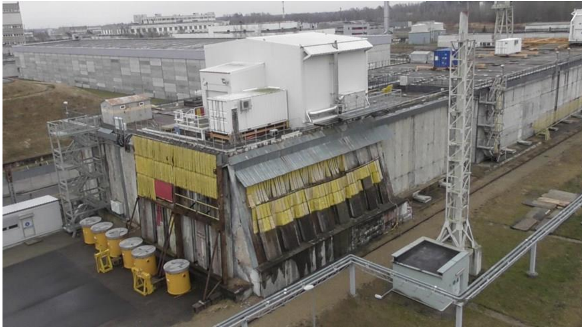
Figure 3.2-7. INPP operational SRW storage building No. 157 with Group G3 SRW retrieval unit RU-3
