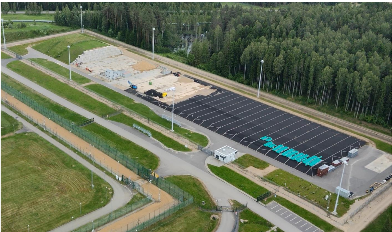
Figure 3-4. VLLW repository module with engineering barriers and a protective wall formed after a particular loading campaign
