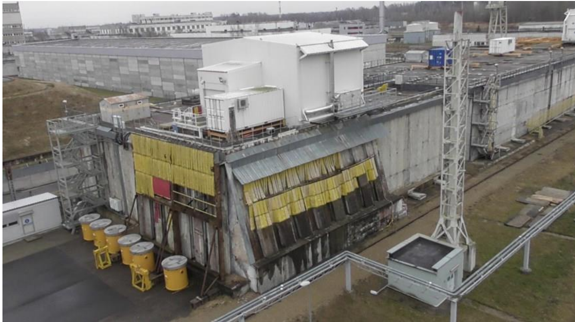
Figure 3-1. Storage Building No. 157 of INPP operational SRW with Group G3 SRW Retrieval Unit RU-3
